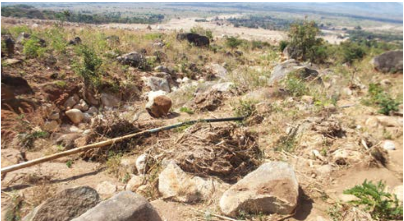
Exposed and damaged water reticulation system at Chitokolo village in Phalombe
